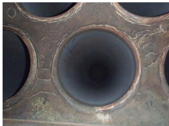
Pic 10: Gas side tubes plate and ends
