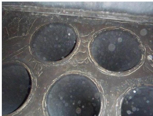
Pic no 8: Looking the pin tubes from the uptake space, all are in good condition including the top tube plate.
