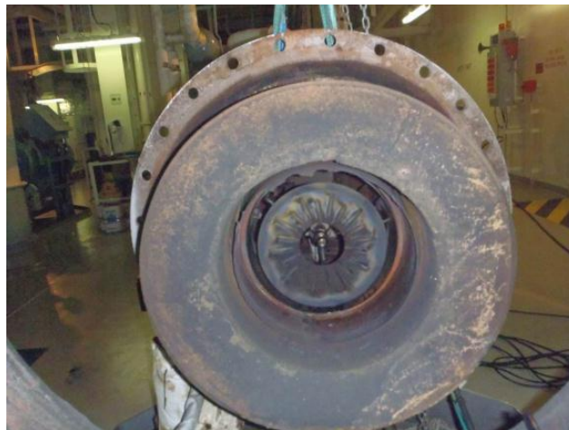
Pic 15: Burner assembly-diffuser plate, vanes, nozzle found in sound condition, the refractory as well is good.
