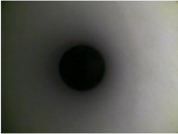
Pic 28: Tube 044- Soot and carbon build up
