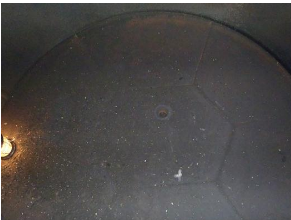
Pic 11: Furnace floor refractory still intact with drain plug
