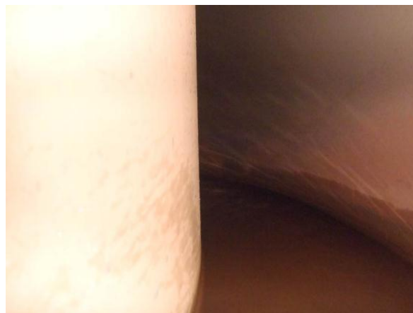
Pic no 13: Showing the bottom ring plate & furnace shell water side. No internal corrosion and negligible loose debris at the bottom
