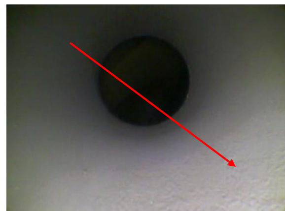
Pic 27: Tube 035- Heavy build-up of soot
