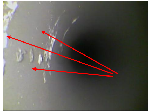
Pic 17: Tube 019- Slight scaling seen
