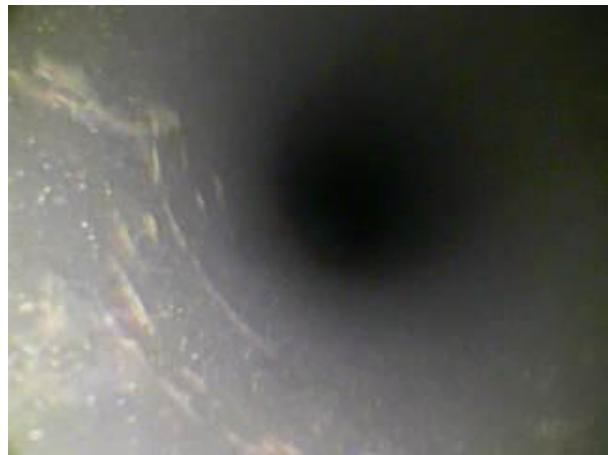
Pic 2: Tube 004- show minor scaling
