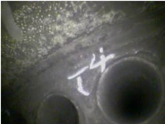
Pic 7: Tube 004- tube plate in acceptable condition
