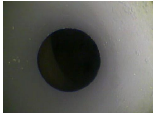
Pic 29: Tube 056- Soot & Carbon build up con't
