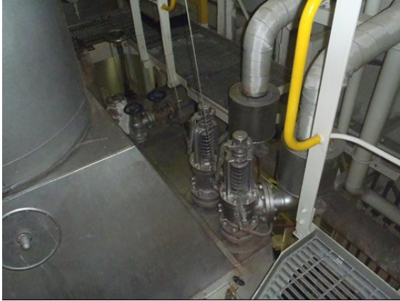
Pic 7: Safety valves
