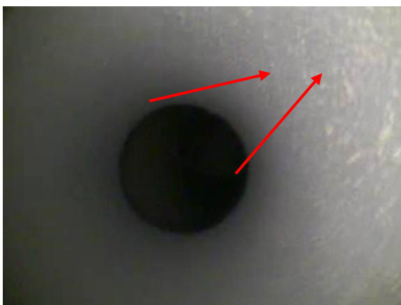
Pic 5: Tube 044- Showing carbon deposits
